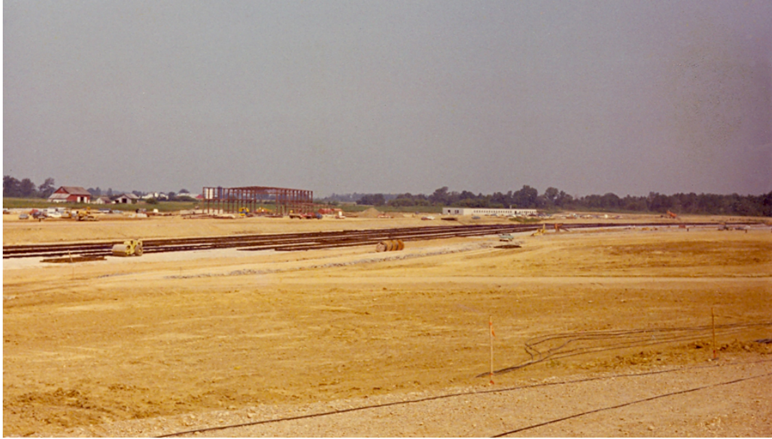
The steel frame for the diesel service & repair shop with the crew's locker & service building to the right.
